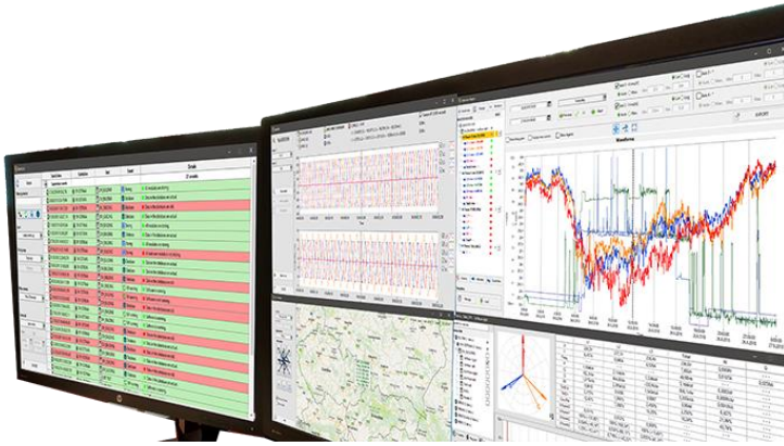
Figure 22: SCADA System ENA SCADA for the control room
