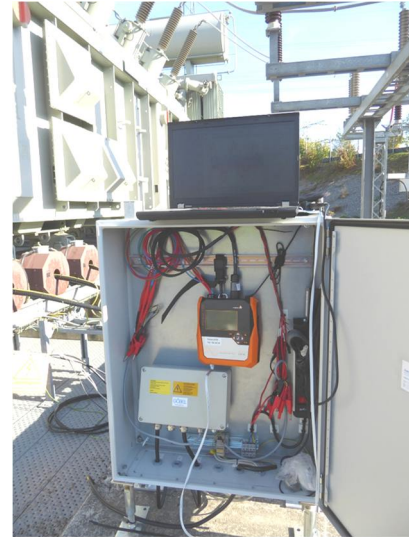
Fig. 4. View of the cubicle installed closed to the transformer, where the PQ device was installed
