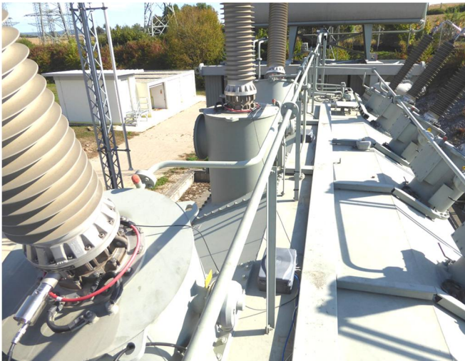
Fig. 3. View of coupling unit connected to the measurement tap of the bushing for the voltage measurement and view of the rogowski-coil used for current measurement
