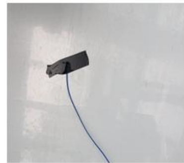
Thermal couple on the back of photovoltaic module
